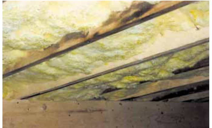
Photograph 1: Icky Crawlspace —Note the condensation on the underside of the fiberglass insulation and the rot at the exposed portions of the crawlspace floor joists.
