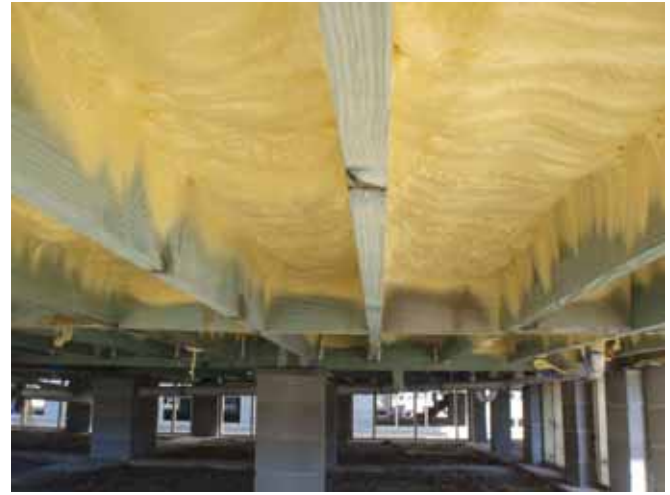
Photograph 6: Spray Foam Between Joists —Floor framing is not completely encased with spray foam in this application. Works only where the crawlspace is open to the outside.
