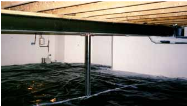
Photograph 5: Conditioned Crawlspace —The way all crawlspaces should look. Dry, warm, part of the house, not part of the outside or part of the ground. Insulated on the perimeter not in the floor. Beautiful.
