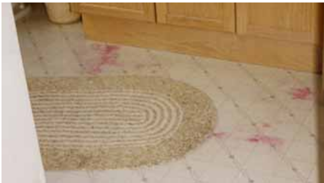
Photograph 4: Vinyl Flooring —Pink spots due to moisture problems arising from the impermeability of the vinyl flooring and ventilated and insulated crawlspace underneath.
